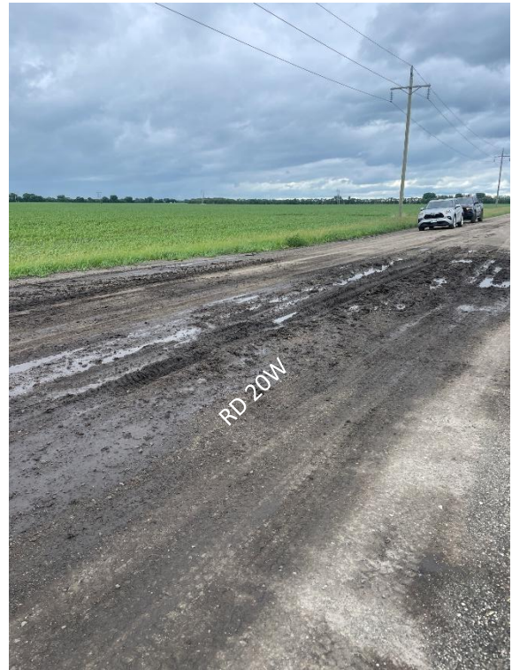
Figure 1009. Rutting in N problem area
